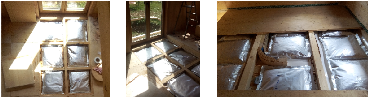
Fig. 4: Macroencapsulated PCM integrated in the floor compartments (left, middle) and in the intermediate ceiling (right).
